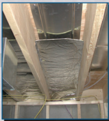
Beneath Radiant Floor
