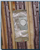
Behind Recessed Lights
